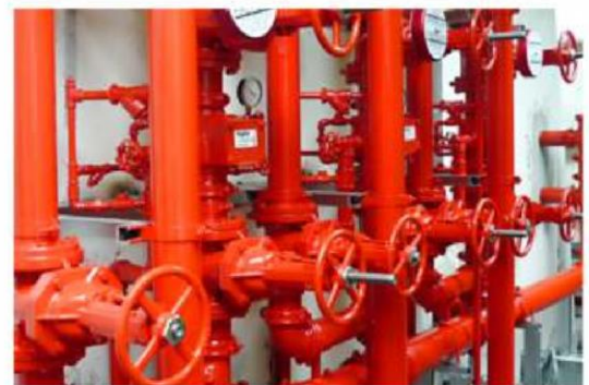
a structure for Application - Fire Fighting
