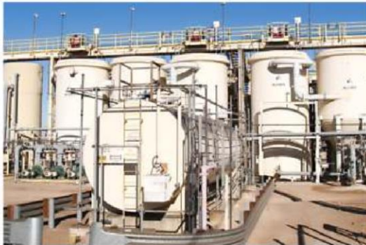
a structure for Application - Reaction Tank
