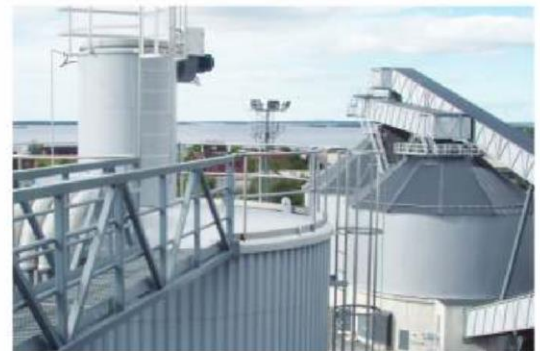
a structure for Application - Ash Handling Plant
