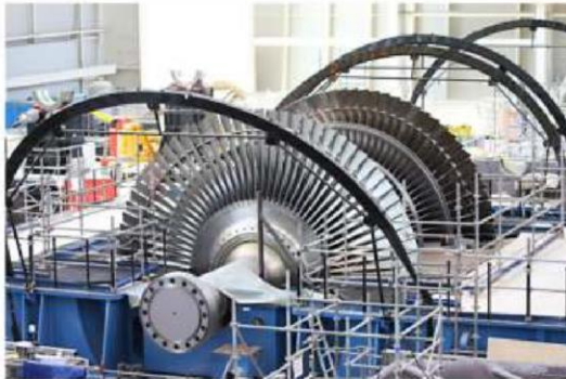
a structure for Application - Steam Turbine
